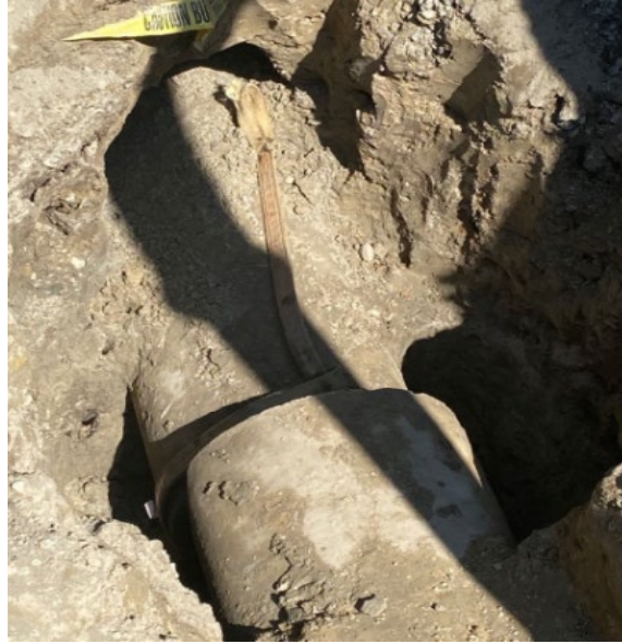
Figure 2: Difference in pipe elevation where collapse occurred
