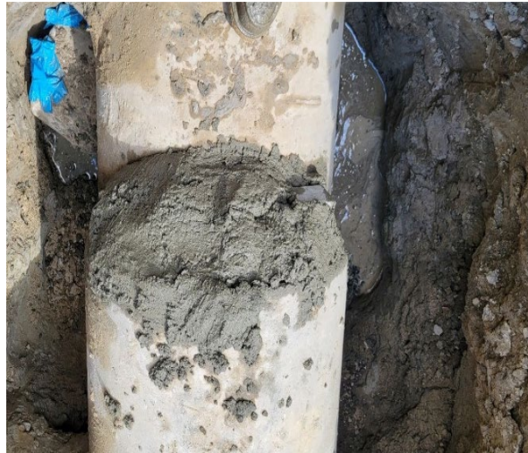
Figure 3: Joint temporarily patched
