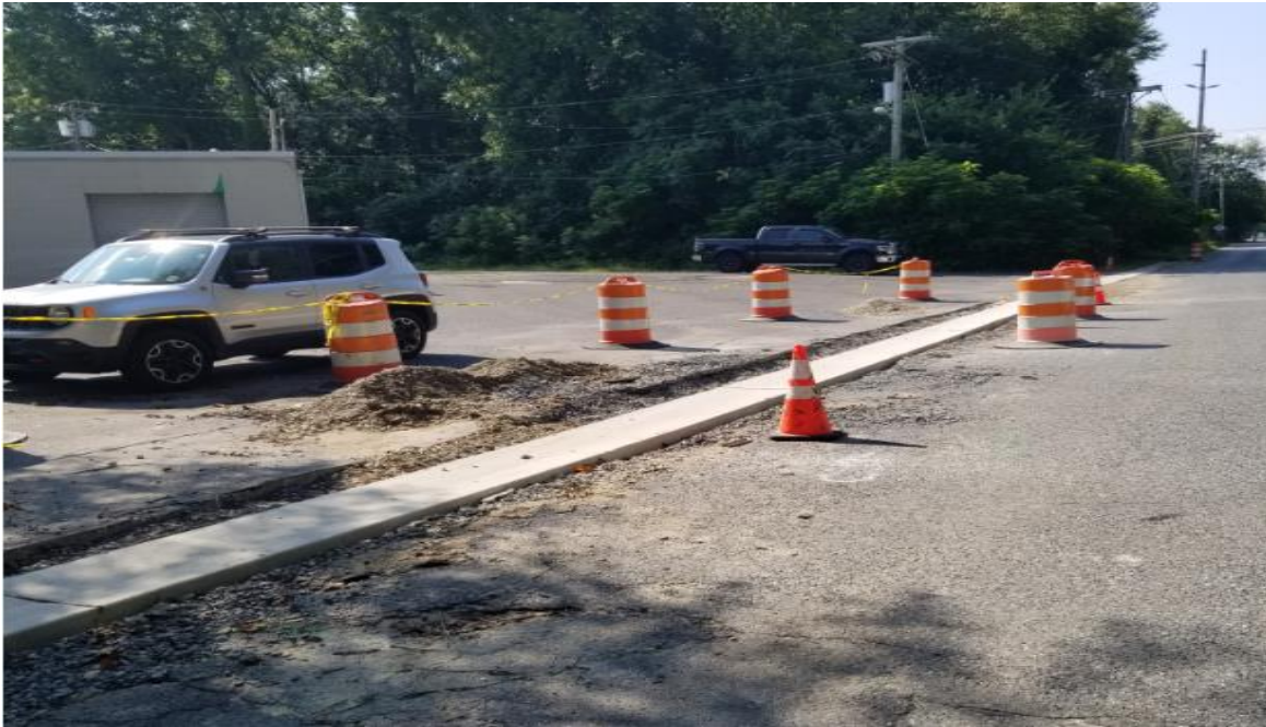
Figure: 2 – Concrete gutter on N. Park drive near Auto Car wash driveway
