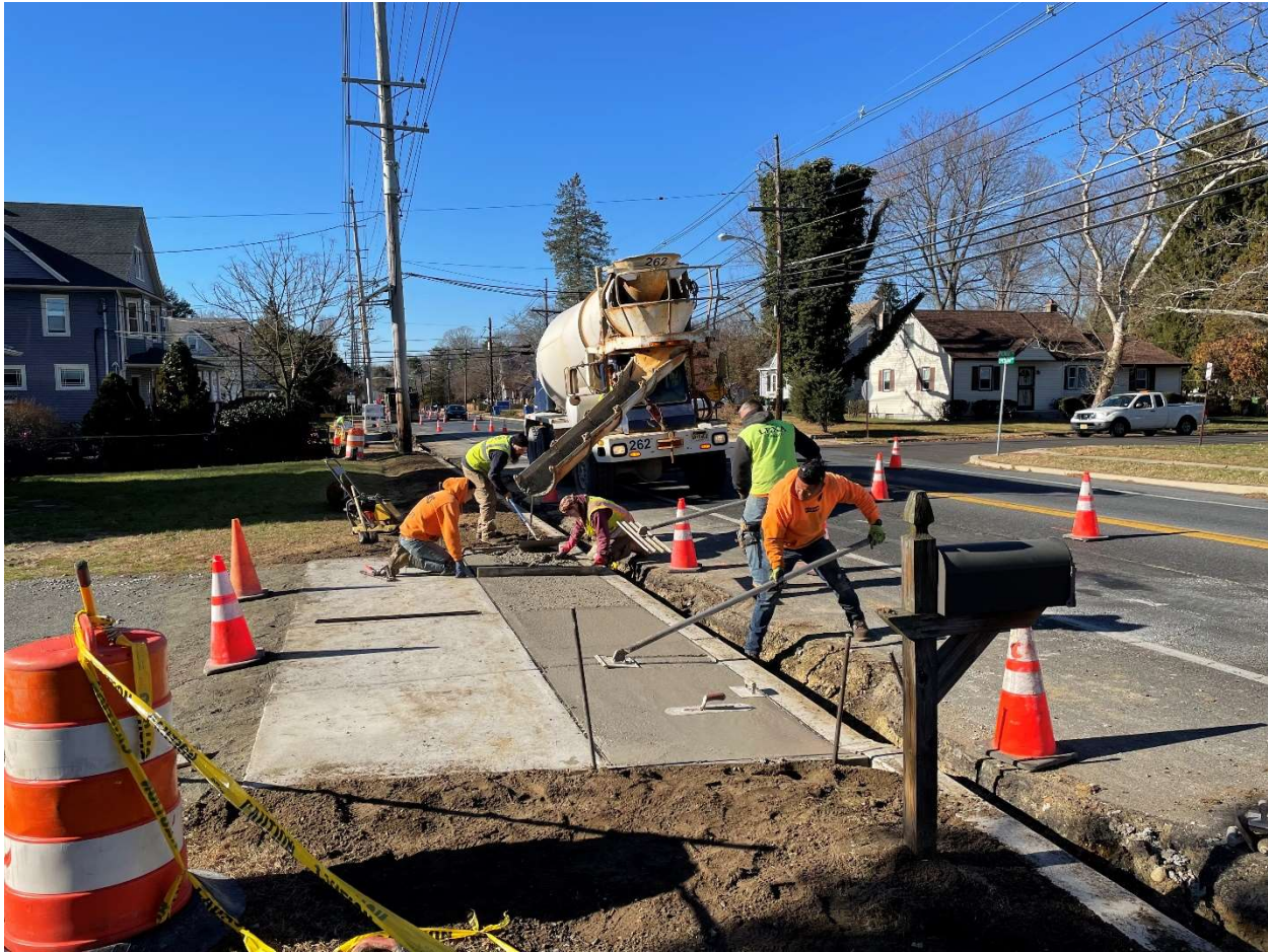
Image 2 – At 125 Evesham Road, Lexa Concrete pours and completes work on new 6” thick concrete driveway. After laborers spread and level the material to the proper grade before striking off and removing excess, the concrete is being float finished perpendicular to the curb.
