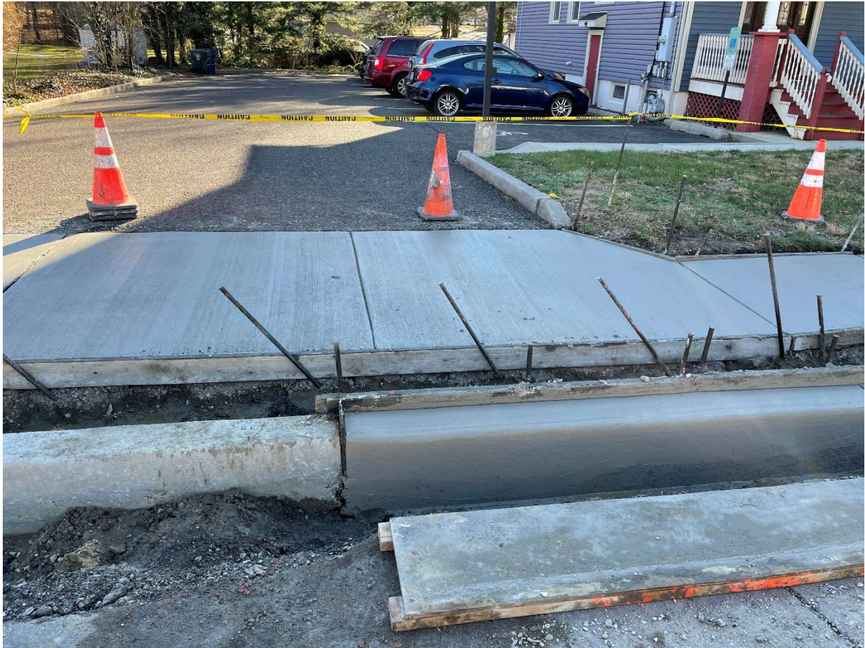
Image 3 – Formwork is removed from recently set new 9” x 18” concrete vertical curb. Following this partial curing, the top of the curb will be finished before being covered with an insulated blanket to provide protection from the weather.
