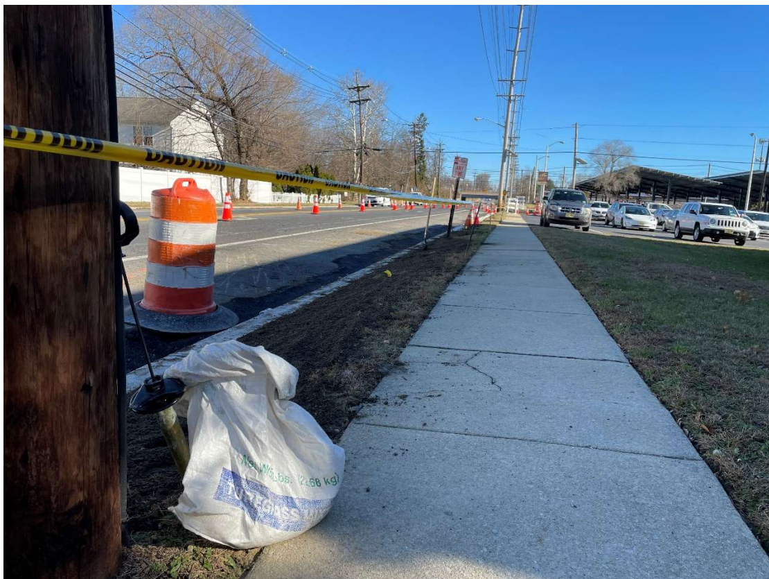
Image 1 – Contractor Lexa Concrete placed topsoil to repair parkway lawn turf along Evesham Road. These areas were recently damaged when existing curb was excavated to begin formwork for new curb.
