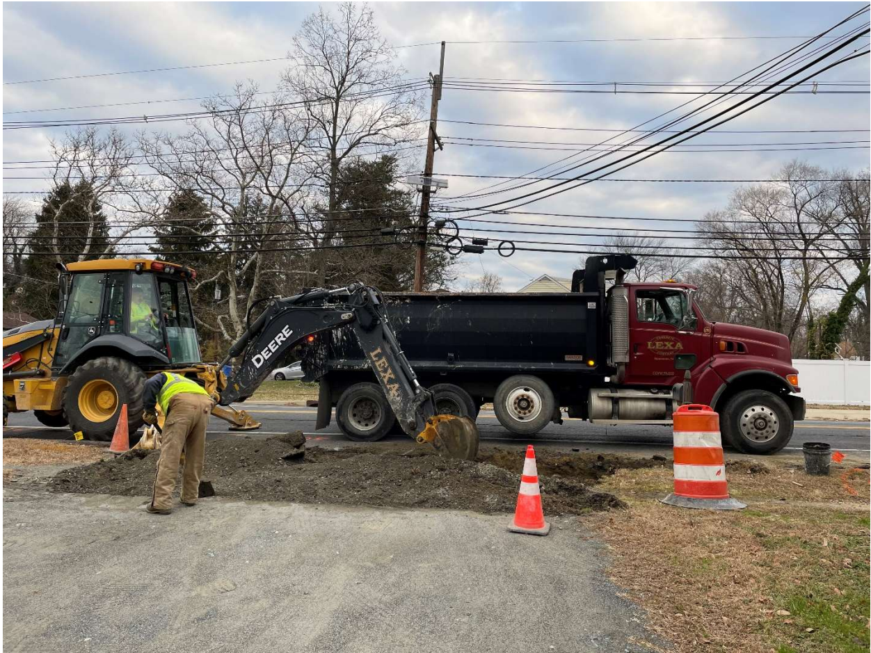
Image 2 – Excavation work taking place to begin construction of new 6” thick reinforced concrete driveway. Existing curb and driveway apron removed in front of 125 W Evesham Road.
