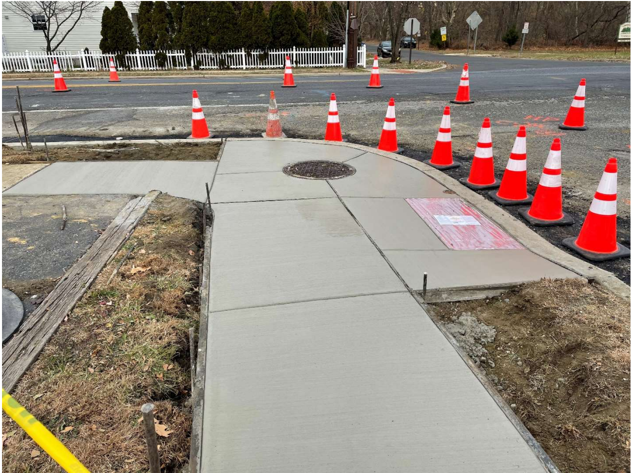
Image 3 – New ADA compliant ramp and sidewalk poured on Friday, 12-10-2021. Pavement adjacent to new curb was repaired using hot mix asphalt and compacted to match existing roadway grade.
