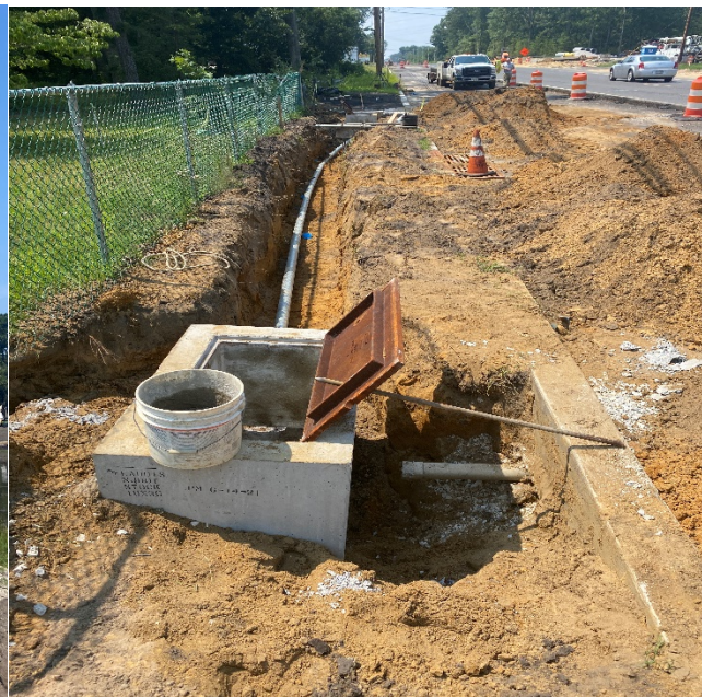
Figure 2: Junction Box/2" RMC Installation
