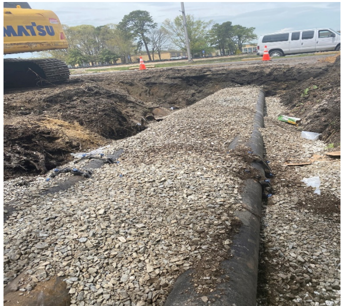
Figure 2: (3) Ductile Iron Pipe Crossing at CCTS
