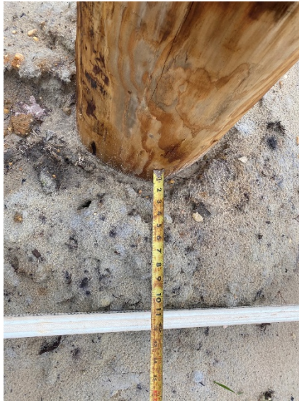
Figure 1: Pole Location from curb
