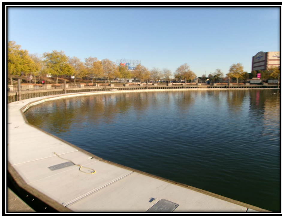
Figure: 3 – Assembly of circular concrete floating dock system at the southern end of the marina
