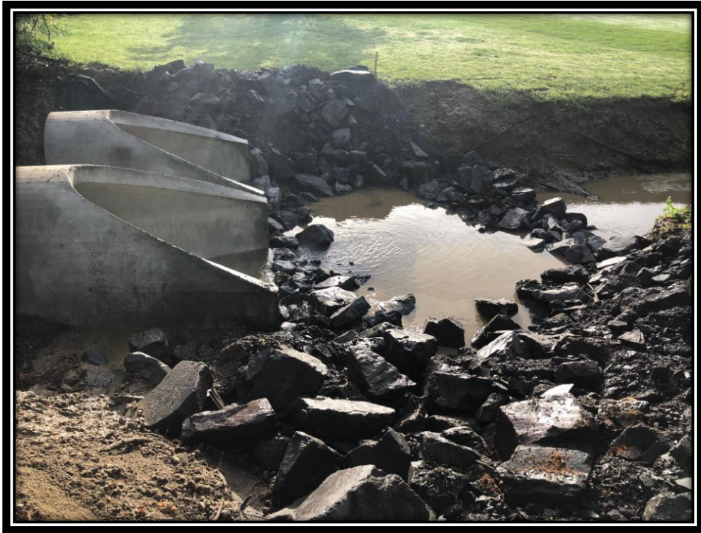
Figure: 2 – Installation of twin 48” concrete flared end sections with rip rap scour hole at the outfall of the twin 48” RCP culvert
