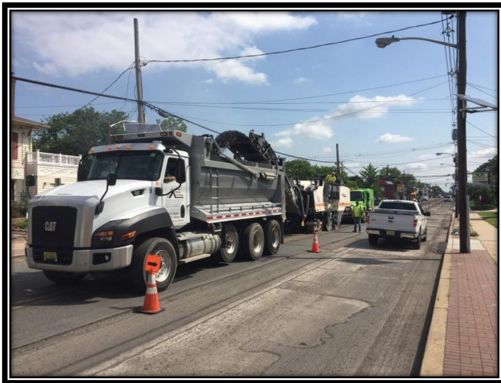
Figure: 1 – HMA milling of the eastbound lane between 42 nd Street and Browning Road
