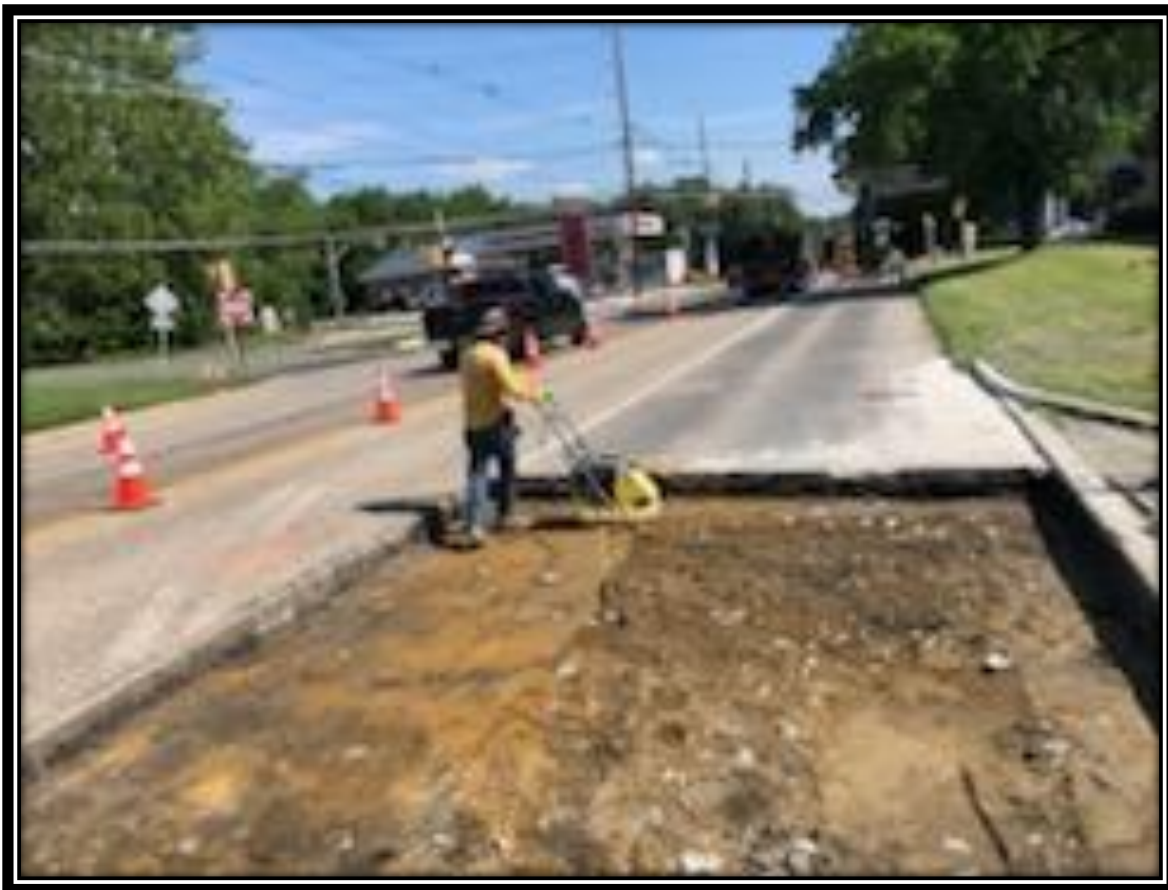
Figure: 1 – Preparation of subbase and reinforcement for the installation of class V, 9” thick concrete slab in the northbound lane between Park Avenue and New York Avenue
