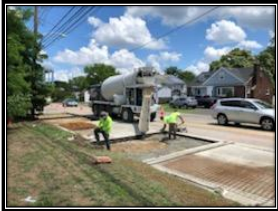
Figure: 2 – Installation of class V, 9” thick concrete slab in the northbound lane between Park Avenue and New York Avenue
