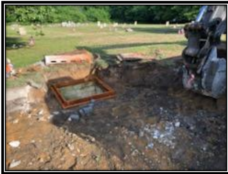
Figure: 3 – Resetting of existing type 'B' inlet in the northbound lane between Park Avenue and New York Avenue
