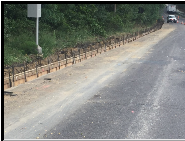
Figure 3: Curb formed on east side of Warwick Road at south side of project.
