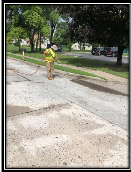
Figure: 2 – Cleaning of existing joints in preparation for sealant installation in the southbound lane between Pleasantview Drive and Erial New Brooklyn Road
